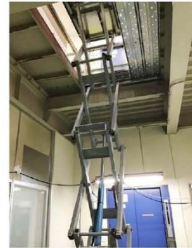
The elevator was malfunctioned and established a temporary elevator.
